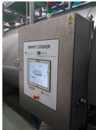
Figure 12. Temperature control system
